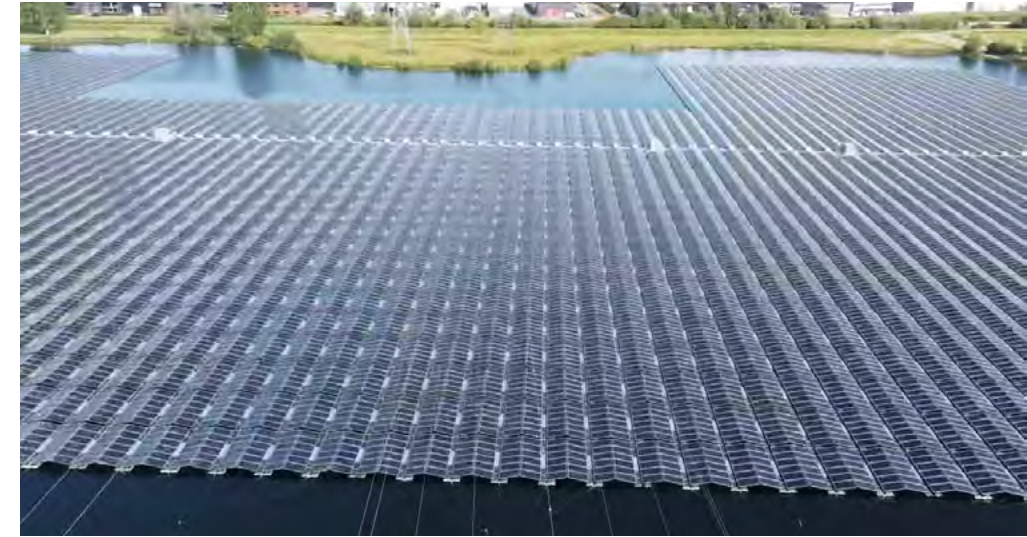
Sekdoorn solar park (15 MW, Netherlands)
